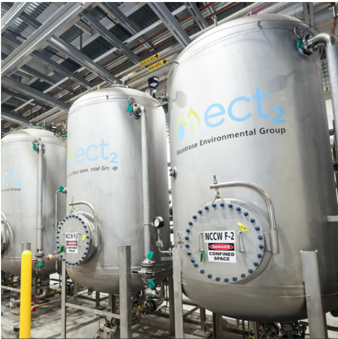
Largest Industrial Wastewater System in the World - Confidential Client
