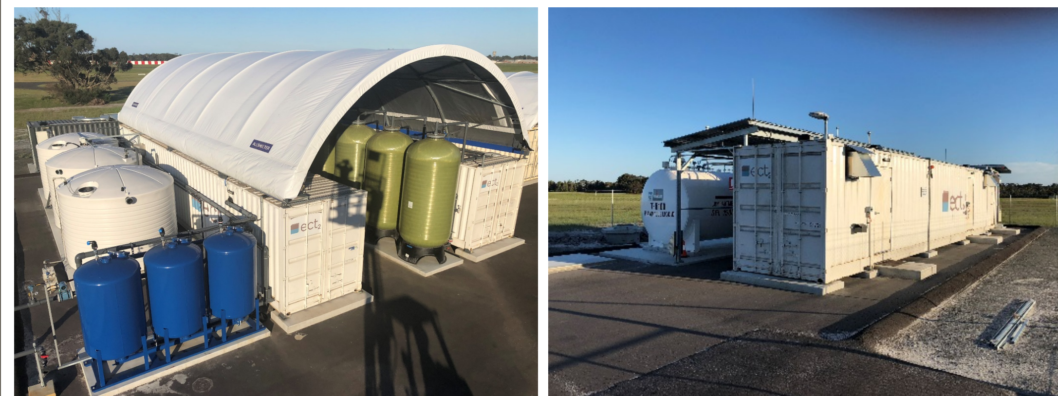
Constructed Treatment System (left) and Centralised Regeneration Facility (right)
